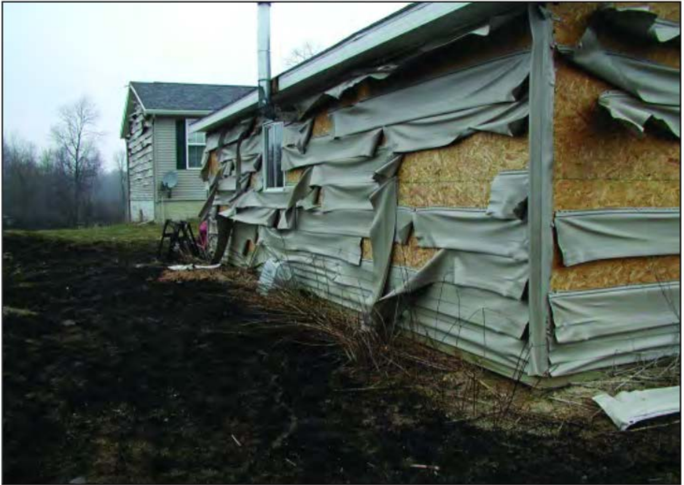
Figure 4 A wildfire in a grassy field melted the siding on this garage and home. (Courtesy of Michigan DNR.)
